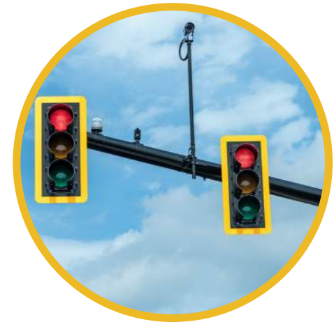
FIGURE 52: UPGRADED TRAFFIC SIGNALS
