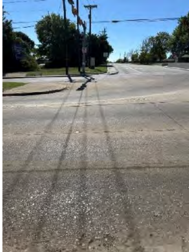
Figure 6. No North-South Crosswalk at Chattey Road
